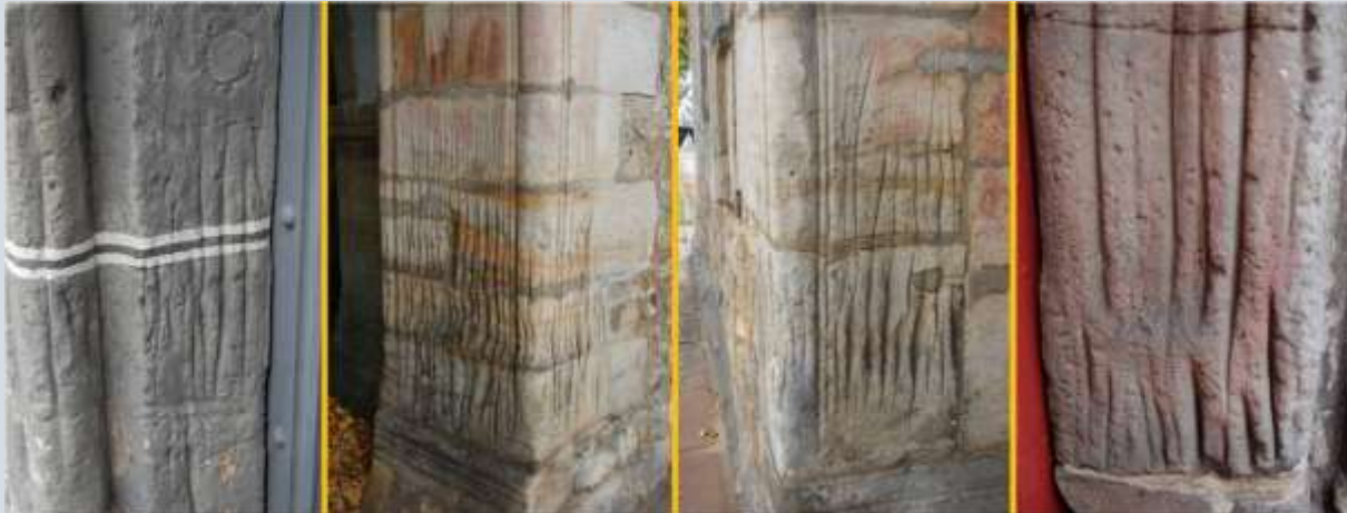
Scratch marks can occur as long, narrow and shallow grooves.
