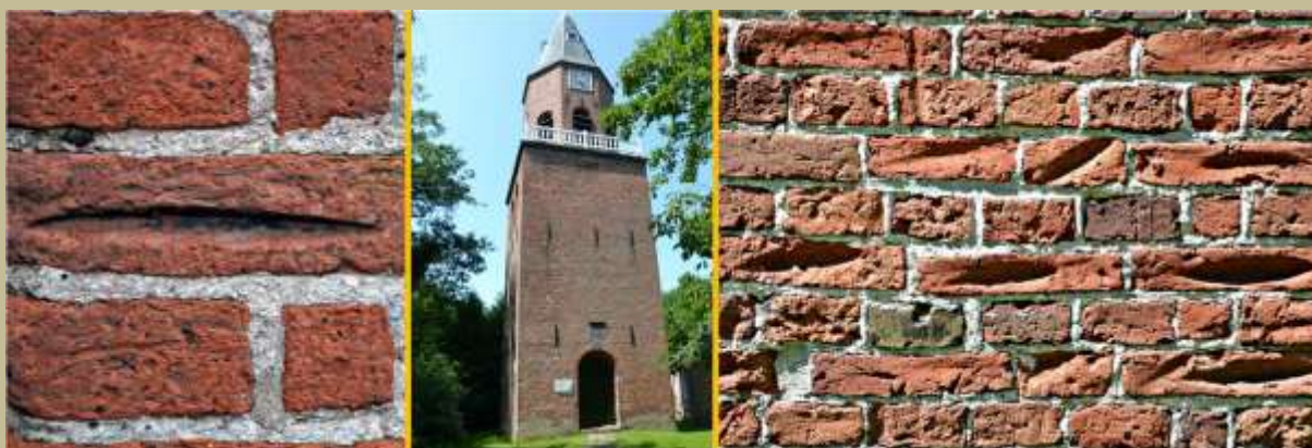
Scratch marks in brick in Wijk bij Duurstede (photo 1) and in Bellingwolde (photo 2+3), in The Netherlands
