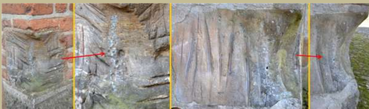
Hollowed out corner stones also belong to the scratch marks
