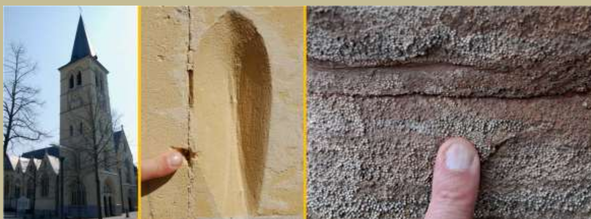
Scratch marks in limestone ('marl') in Bree in Belgium (photo 1+2) and in Rogenstein in Braunschweig in Germany (photo 3)
